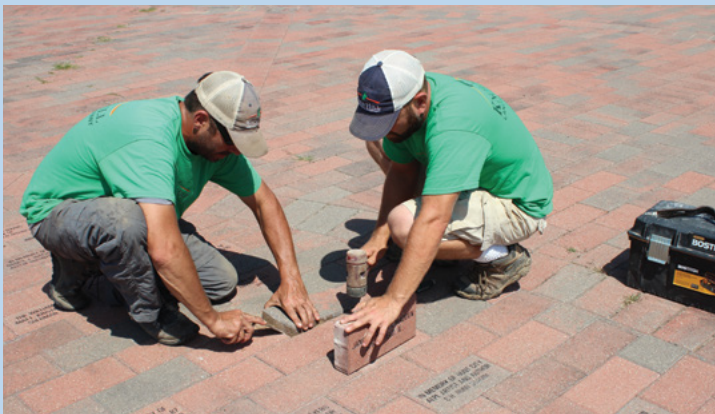
Knob Hill Landscaping staff install Pavers in Union Square Park during the ongoing ALPLF campaign. Knob Hill also generously donated mulch for the park grounds located in Union Square.
